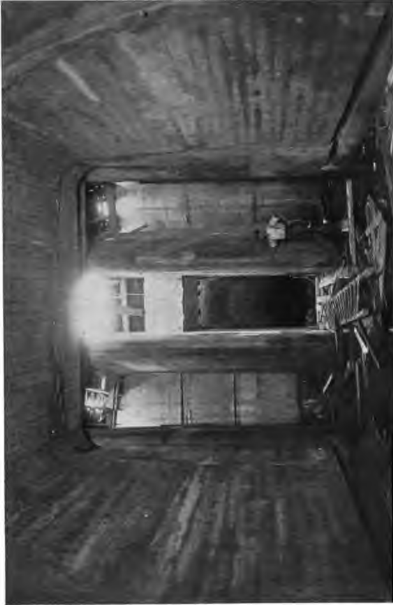
PLATE 155.—Contract 62 or 68. Junction of Cut-and-cover Aqueduct and Steel Pipe Siphon. Central pipe laid and flow into it controlled by sluice gate. Side opening for future outside pipes bulkheaded off.
